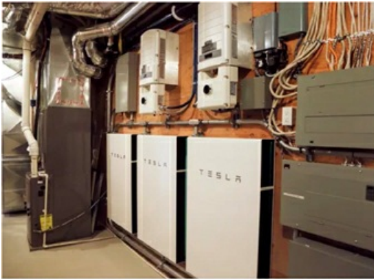
Tesla Powerwall batteries. Andrew Francis Wallace/Toronto Star via Getty Images
